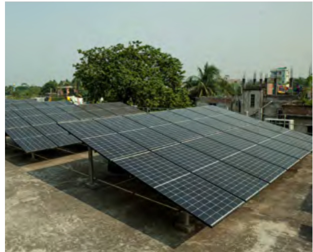
Figure 5: Solar Panels in Multifabs Limited
