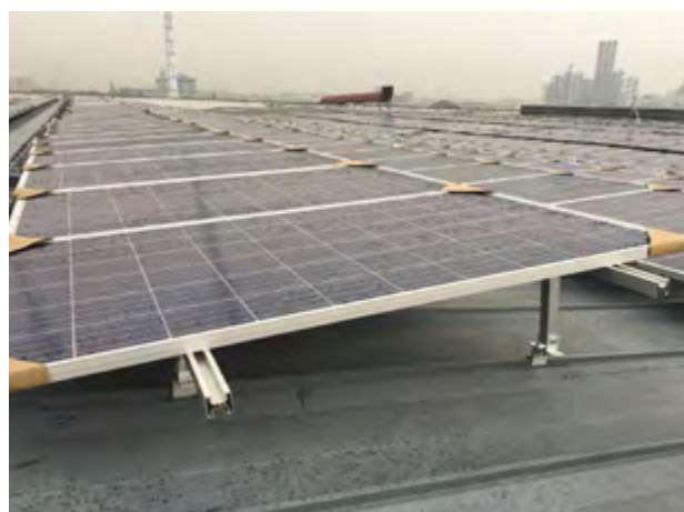
Figure 3: Solar Panels at Tarasima
